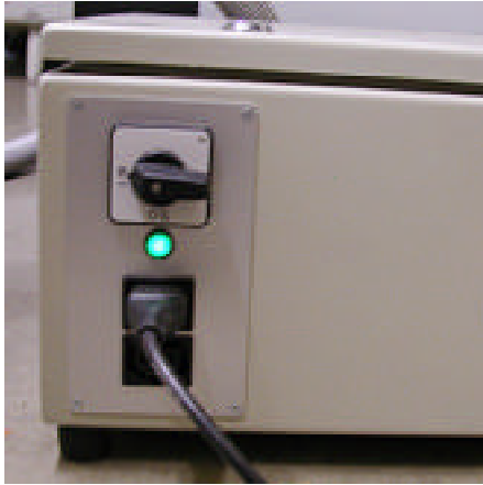
Figure 5: The power box is switched on, as indicated by the green light.
