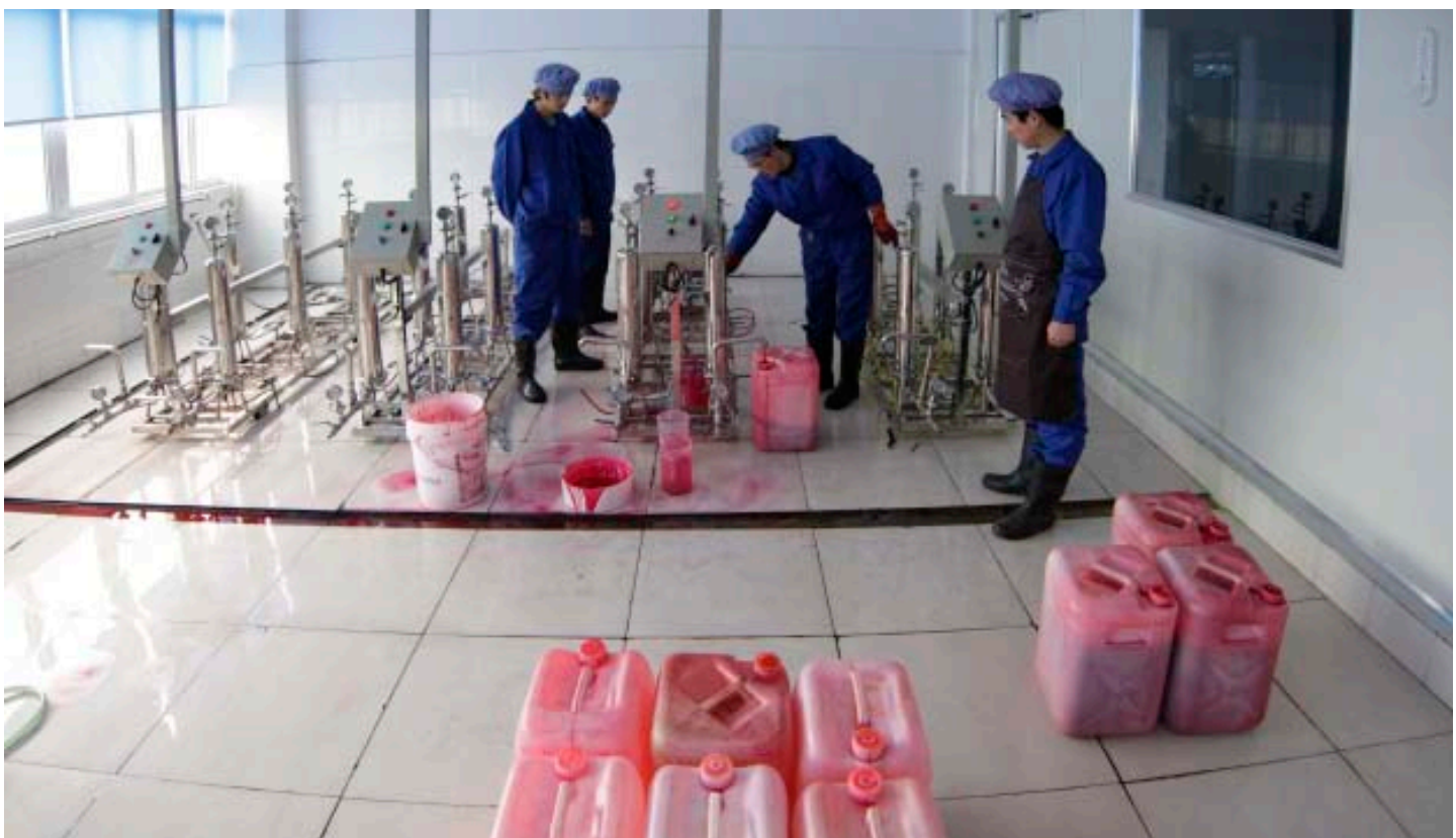
Here you see the newly installed equipment. I spent several days in the new factory, and also visited the old former factory. The new factory is improved in every way, shape, and form. It has considerable amounts of sophisticated equipment on several floors.
