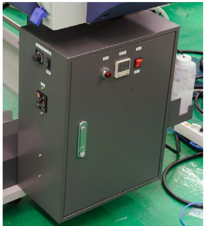
The electronics cabinets are for all the power supply.
