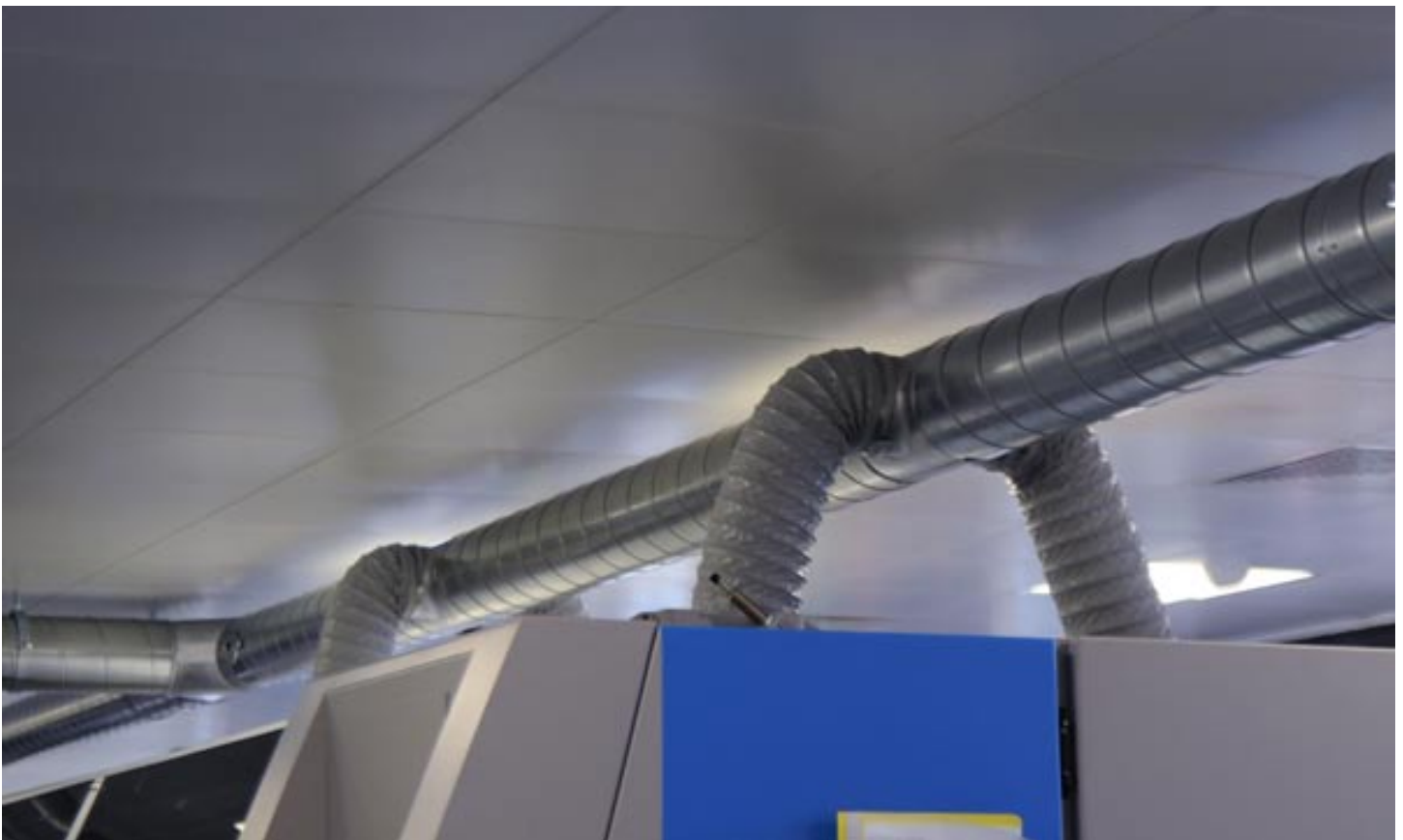
Exhaust tubes are not only to suck the odor and ink mist, but to remove some of the heat too.
