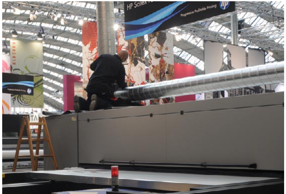
Although UV inks are a lot less harmful than solvent inks, an exhaust system is always recommended to get rid of heat from UV lamps and mist from the inks. In this photo, the exhaust system of the HP Scitex flatbed 6050 being installed at FESPA Amsterdam '09.
