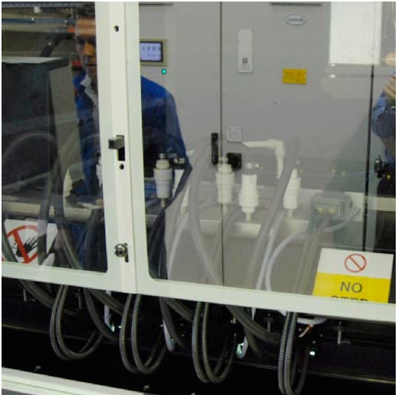
FastJet curing area with the nitrogen blanket, at Sun FastJet Factory.
