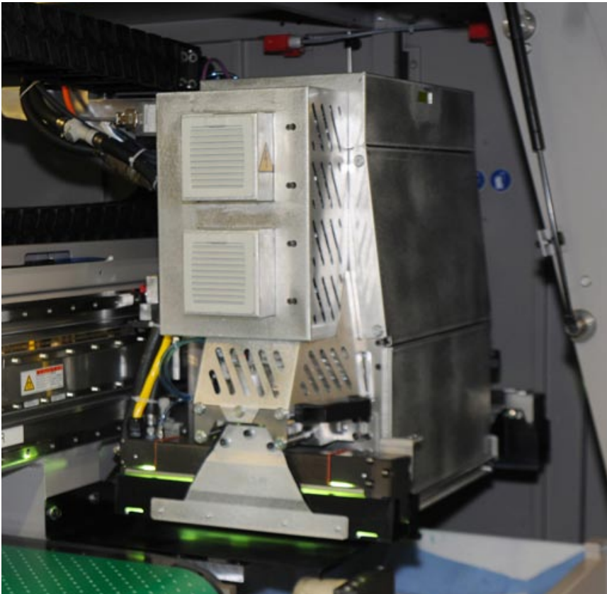
Water-cooling carriage for the UV lamps, at Spuhl factory 08
